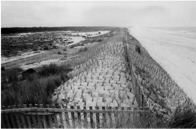
Figure 16. Reconstructed sand dune system in May 2000. To stabilise the sand, revegetation was performed with transplants of Ammophila arenaria .
