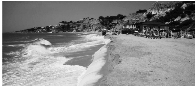
Figure 15. View of the Pine Cliffs beach after artificial sand nourishment. To reduce the amount of sand lost annually, tubes made of geotextile material filled with sand have been used for sand maintenance on the beach.
