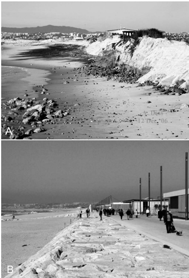
Figure 14. Views of the Costa da Caparica beach deprived of sand in 2006 (A; courtesy of Alveirinho Dias) and the beach and its marginal strip after the last major intervention in 2014 (B). This arrangement has remained substantially constant since 2010, with only some interventions in the support structures and the replacement of small amounts of sand that are lost annually (a few hundred thousand cubic metres per year from approximately 2 km of beach).
